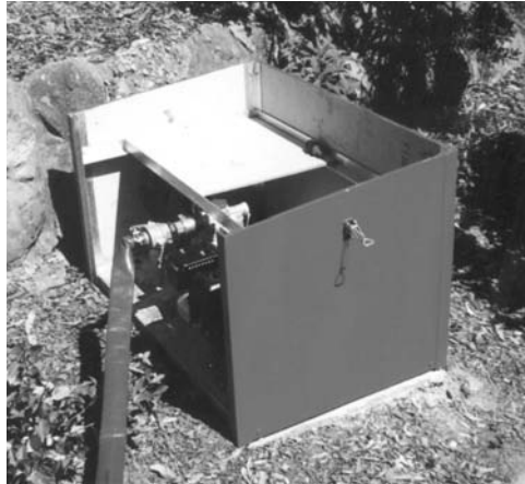
PROTECT YOUR PUMP FROM FIRE
